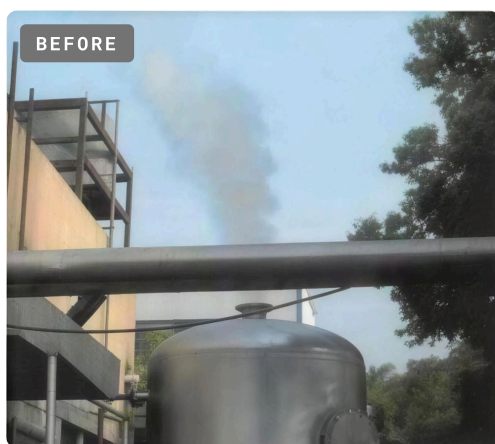
Flash steam venting to atmosphere above the condensate tank.
