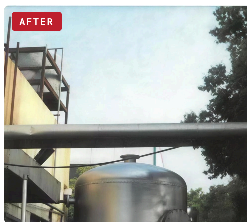
No plume: the flash steam is now reused.
