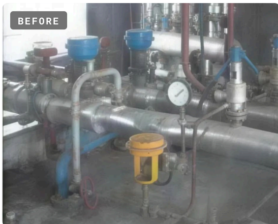
Control-valve stations on the steam main.
